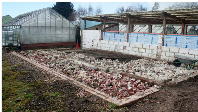
30 March After clearing by Network Rail group and partial infilling with rubble.
