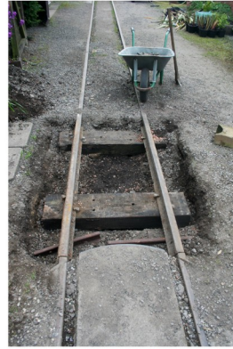
After digging out the old sleeper, two new sleepers were put in and rotated until under the rails. Two short lengths of rail were used to raise the height of the rails nearest to the camera. The left rail furthest from the camera is held down with the standard gauge bolts, the remaining fixings are narrow gauge spikes. All that remains to do is push ballast under the sleeper and fill in and tamp the hole.
