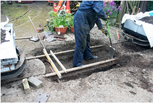
Digging out the old sleeper. At the left hand side of the hole is a spirit level, on its right is gauging stick to ensure the distance between the rails is 600mm.
